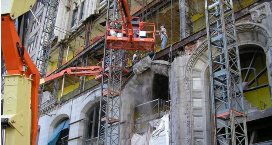
90 West Street's facade was destroyed on 9/11, and its ornate masonry was craftily rebuilt using a combination of old skills and new techniques.
